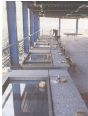
2. Wall panel depot on the floor where the panels will be installed.
